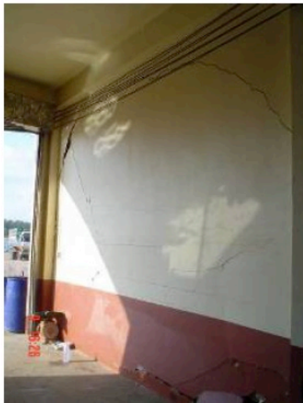
(a) Cracks on a wall
