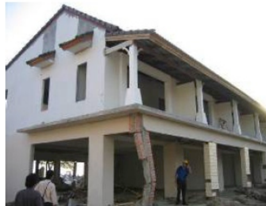
(b) Bending failure of column
