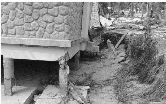
(a) Foundation failure
