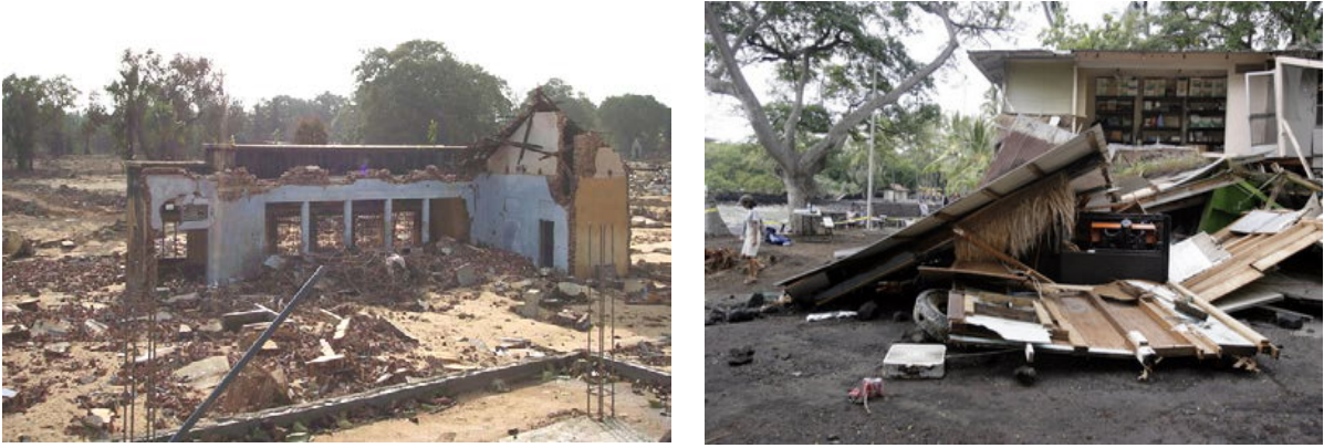
Figure 6.12 Damage Level 3 (Collapse) for non-solid building
